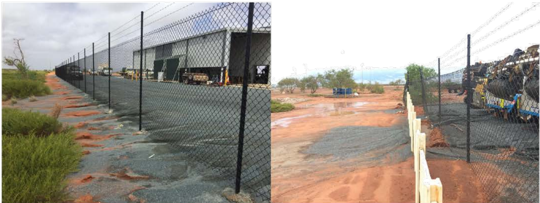
Figure 2: Yards have eroded onto neighbouring land from inadequate use of materials for surface treatments (fines - cracker dust), incorrect grading and no infiltration measures (left Kingsford Smith, right Wedgefield).
