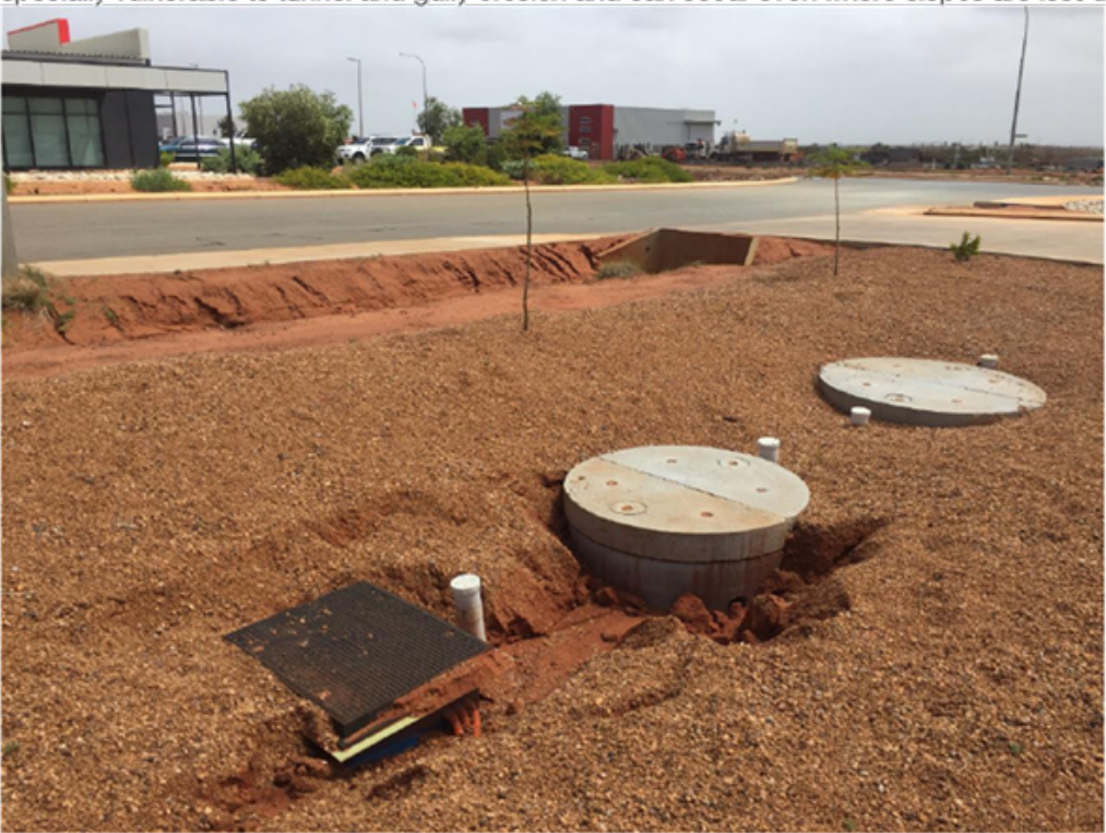
An example of tunnel erosion around the concrete lids in Kingsford Smith
