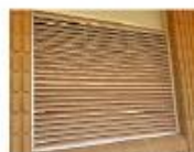
Fresh Air Intake
