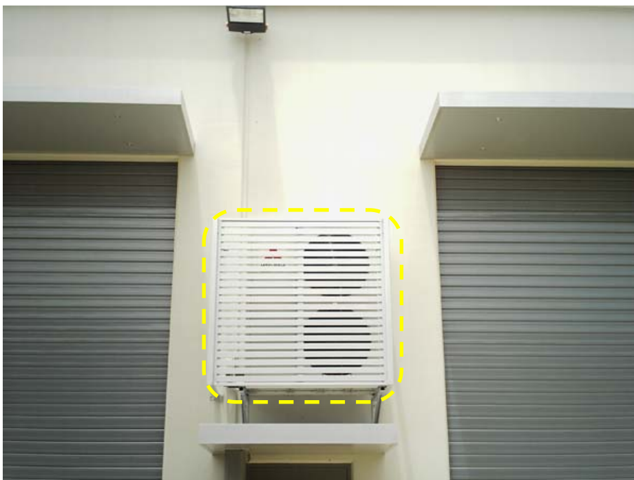
Requirement in Scenario B, C, D, G, H & I – screened air conditioning units
