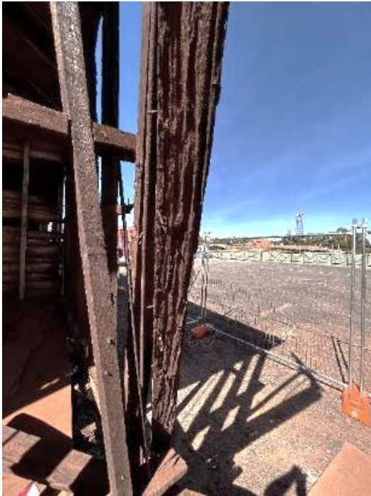
Figure 82: Termite damaged verandah timbers
