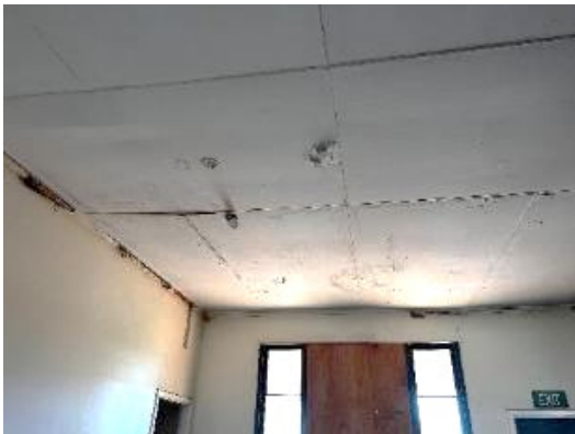
Figure 87: Damaged ceiling in Main Hall 1
