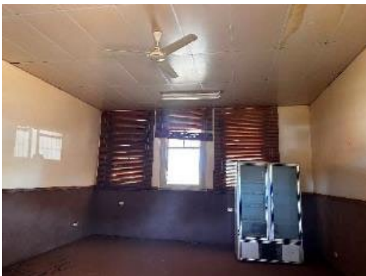
Figure 88: Damaged ceiling in Main Hall 2
