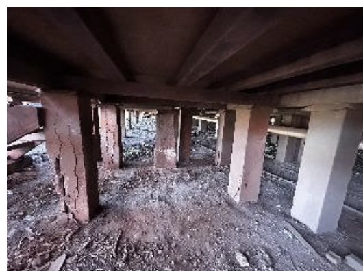
Figure 76: Damaged and replaced concrete stumps
