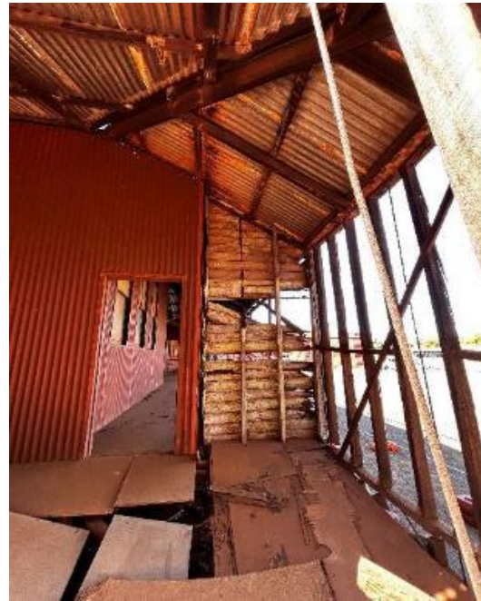
Figure 69: Collapsed verandah and loss of cladding materials
