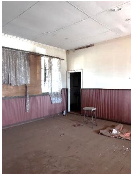
Figure 85: Boarded up window and damaged ceiling
