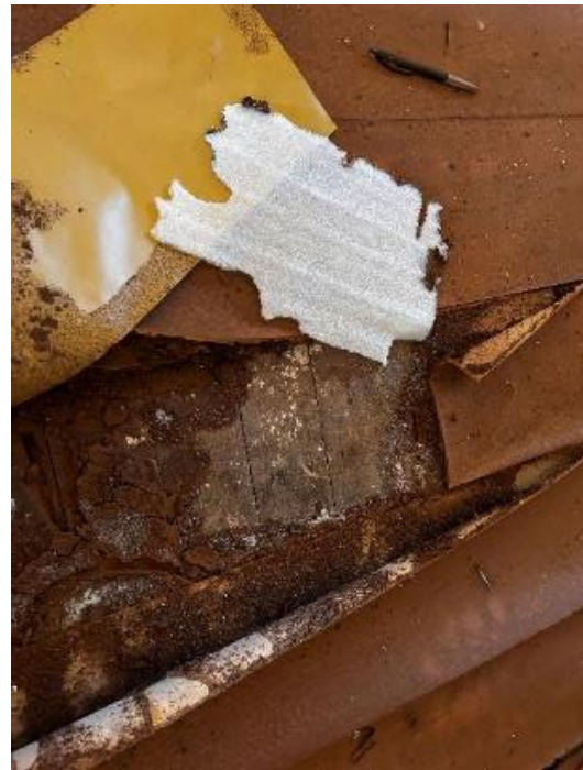
Figure 89: Damaged timber floor in Main Hall 2
