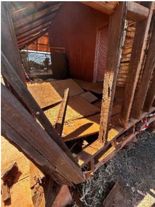
Figure 68: Collapsed northern verandah
