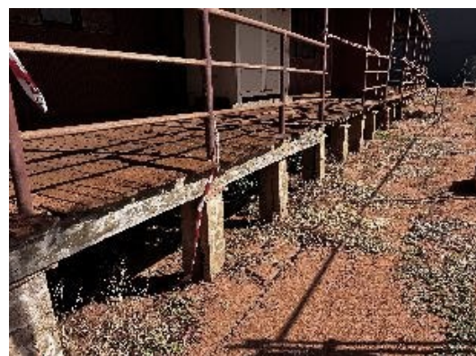
Figure 75: Verandah in poor condition
