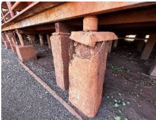
Figure 66: Typical concrete damage to stumps
