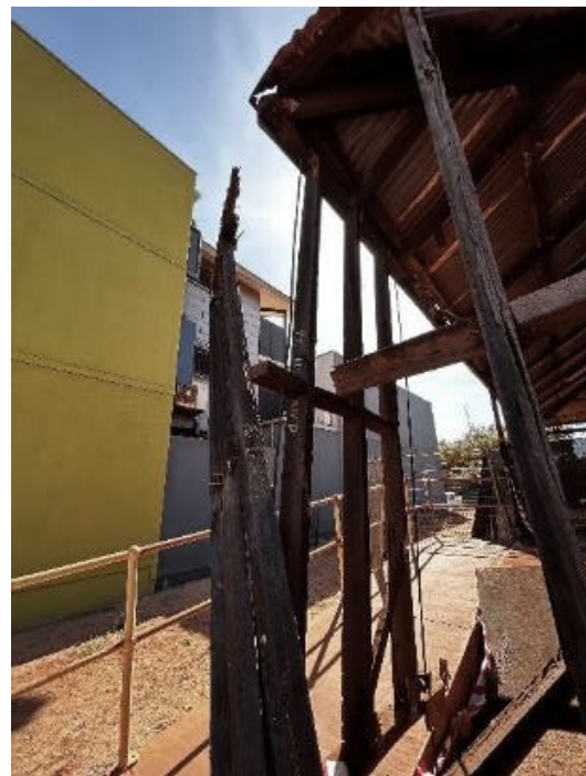
Figure 70: Damaged verandah timbers
