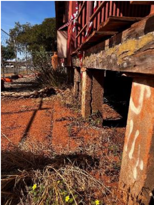
Figure 78: Damaged stumps and verandah facing plate
