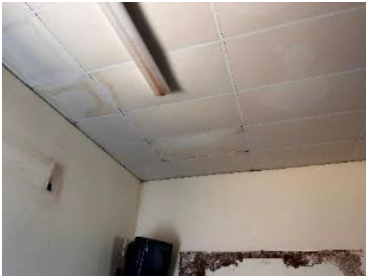
Figure 91: Damaged suspended ceiling in Main Hall 2
