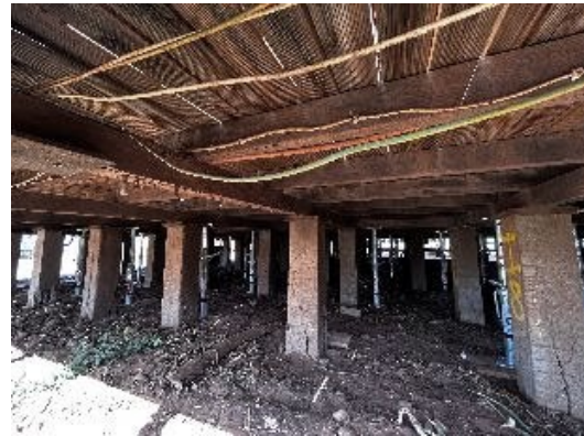
Figure 74: Unsafe wiring under the building
