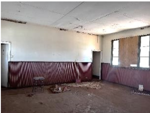
Figure 83: Damaged ceiling in Main Hall 1
