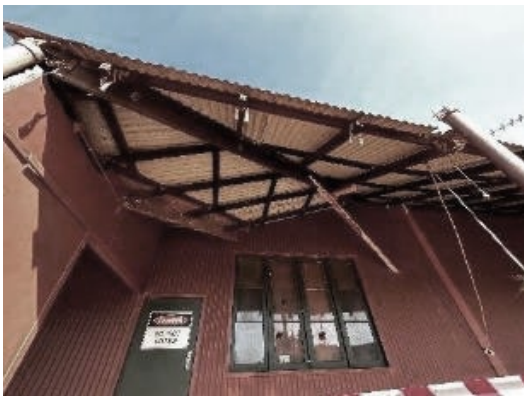
Figure 73: Damaged verandah canopy timbers
