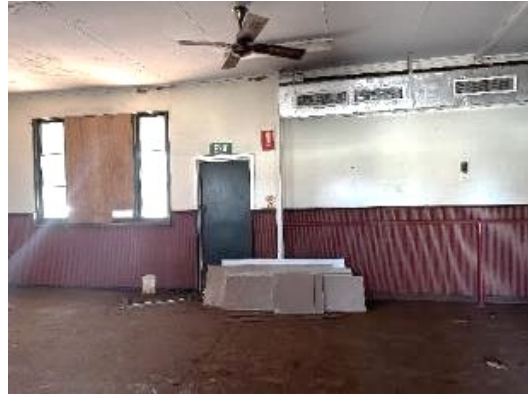
Figure 84: Boarded up windows and loss of wall cladding
