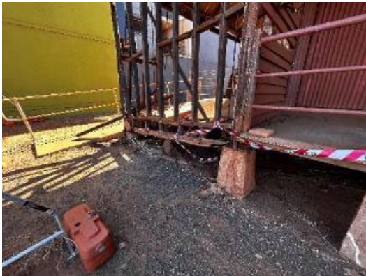
Figure 67: Collapsed northern verandah
