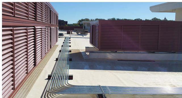
Locating noise generating services such as air conditioners on roof areas reduces the visual impact on the streetscape.
