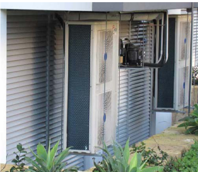
Air conditioning units located discretely and away from public view, if not located on the roof of the building.
